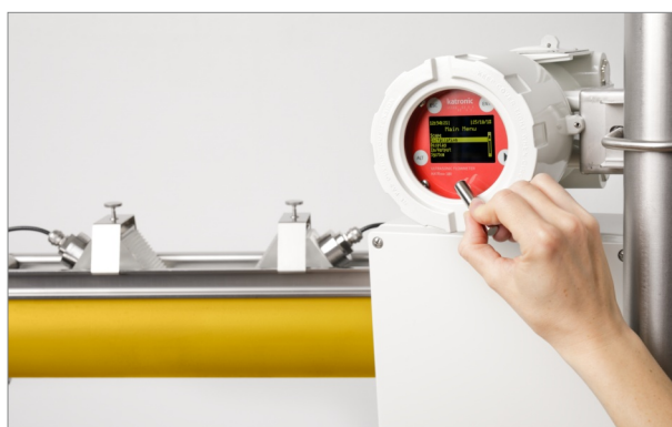
KATflow 180 and G5 type transducers in operation
